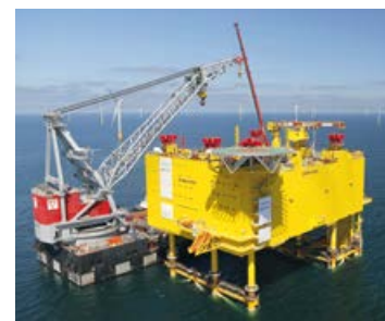
Converter platform for wind farm SylWin1, where the alternating current generated by the wind turbines is converted into direct current and transmitted onshore by sea cable with low power loss
